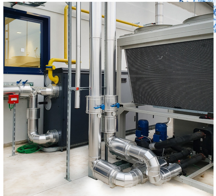
HVAC plant exterior pipework
