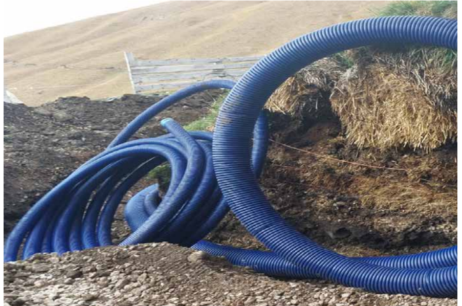
General view of the installation
