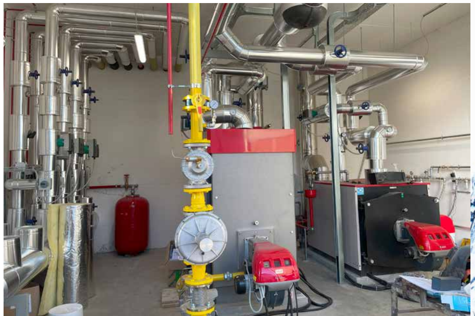
An overview of the plant
